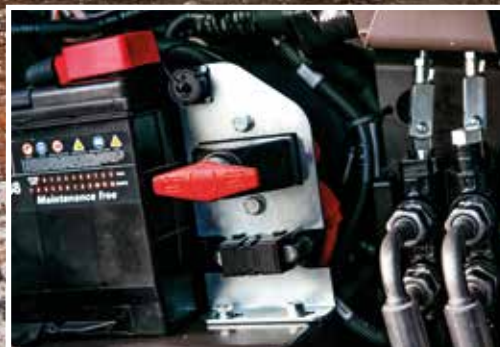
Battery disconnect switch for easy maintenance.
