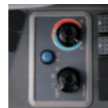
A/C Control Panel
